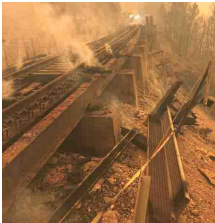
Damaged bridge near Moccasin, Calif. – July 25, 2021. Nearby BNSF Gateway Subdivision (ex-WP “Northern Extension”) siding at Moccasin, Calif, is 6.0 miles north of Keddie, Calif., at BNSF MP 196.8 measured south from MP 0.0 - Bieber Line Jct, Oregon. Bieber Line Jct. is the main track connection within Klamath Falls, Oregon, between BNSF ex-GN Klamath Division, and UP ex-SP Oregon Division main line (Photo Courtesy of BNSF)
