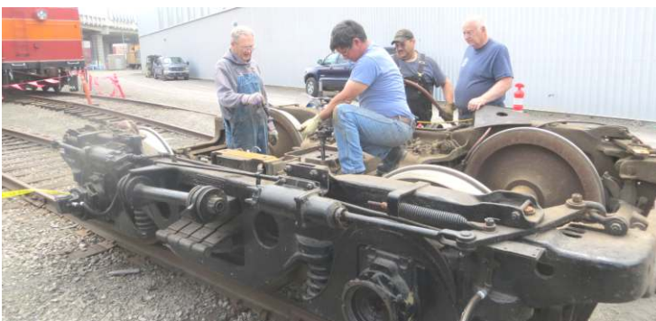
Round End observation car B truck repairs being accomplished June 23, 2019. left to right: Bob Slover, Wayne Yetter, Bob Frazier, and Doyle McCormack. Photo by Arlen Sheldrake.
