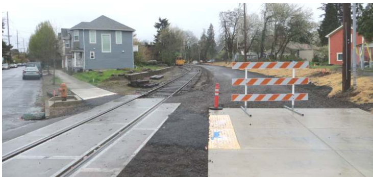
Springwater Trail Gap, SE Umatilla to SE 13 th Avenue construction is underway with this new segment next to the Oregon Pacific Railroad targeted to be completed by July 1, 2019. Photo by Arlen 4/8/2019.
