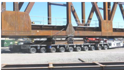
Drano Lake BNSF Bridge Replacement ready to be Moved near Mitchell Point
