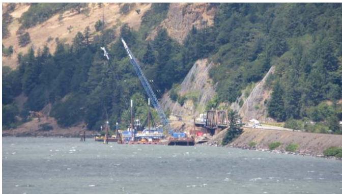
Drano Lake BNSF bridge replacement Construction from Mitchell Point ymuseum.org , is located at 300 East Port Marina Drive.
