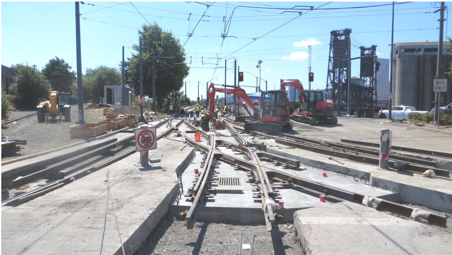
New MAX track work being laid onto the Steel Bridge Eastern Entrance Ramp - Photo by Arlen Sheldrake on August 18, 2020
