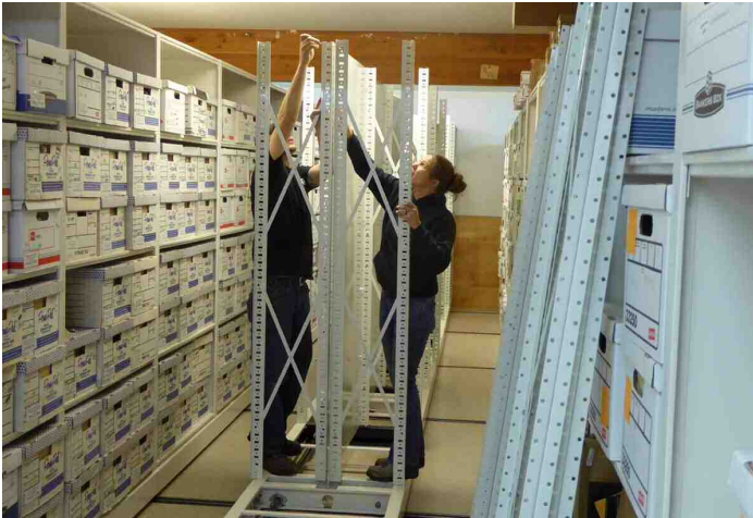
The contractor's crew installs the Borroughs carriage of mobile shelving on the west side of the lower floor.
