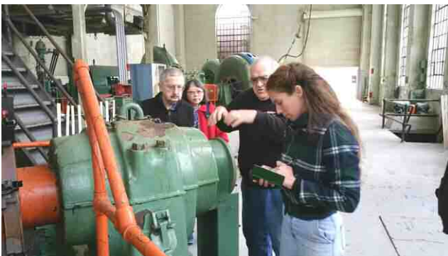
Tour Guide Claire talking with George Hickok, Bill Markwart and Midori Suzuki in the Generator Room.
